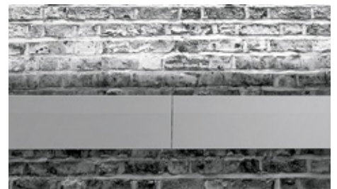
Single mounting or linear compositions with a minimum distance between modules of 5mm.
